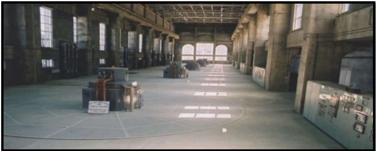
[fig.Canal Head Power House (CHPH)]
